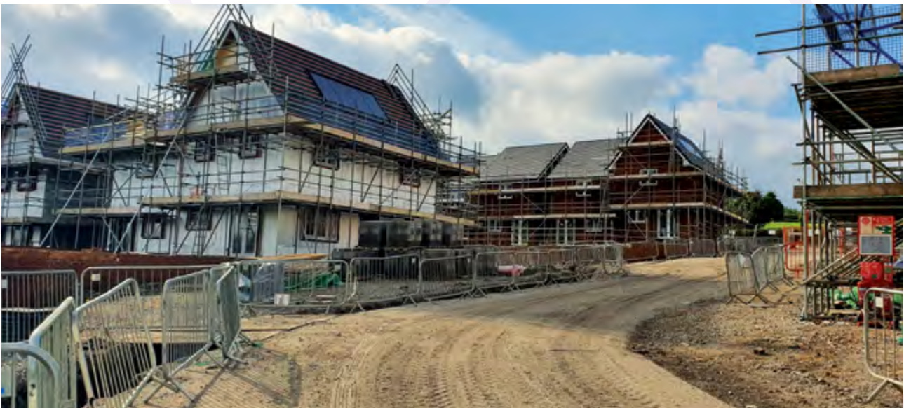
Construction in progress at an affordable housing development on the former Penallta Colliery site (UWHA)
