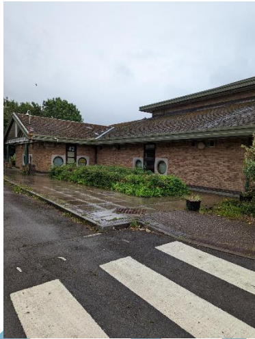
Figure 19 – Western aspect of the building (area of roof to be affected by the works).
