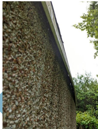
Figure 24 - Gaps between flat roof and wall of the nursery.
