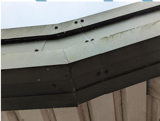
Figure 21 – Gaps under metal fascias and soffits.
