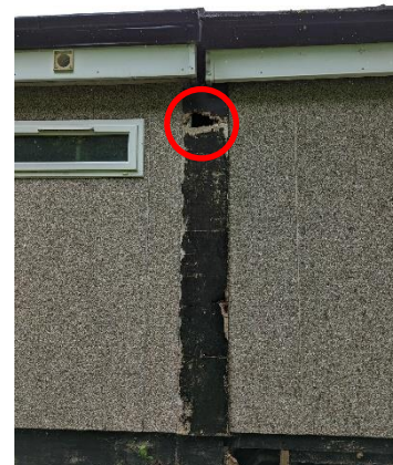
Figure 22 – Gap between the nursery building.
