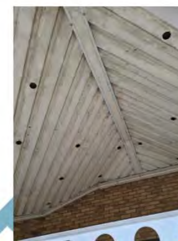
Figure 18 - Ventilation holes under the roof at the main entrance to the building.
