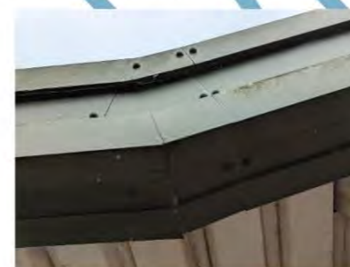
Figure 21 - Gaps under metal fascias and soffits.
