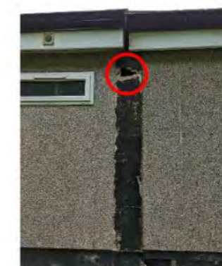
Figure 22 - Gap between the nursery building.
